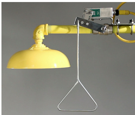
Figure 20: TopWorx Switch Installed on a Safety Shower
